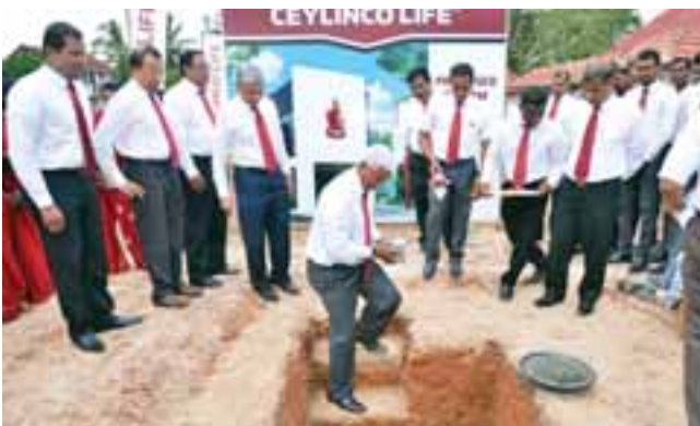
Ceylinco Life has commenced construction of a new eco-friendly building to house its branch in Chilaw, continuing efforts to reduce the company's carbon footprint.
